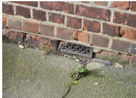
Some repair needed
