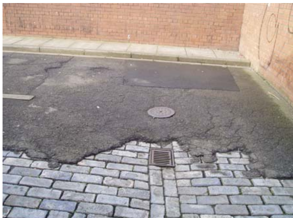
Poor attempt to tarmac the setts
