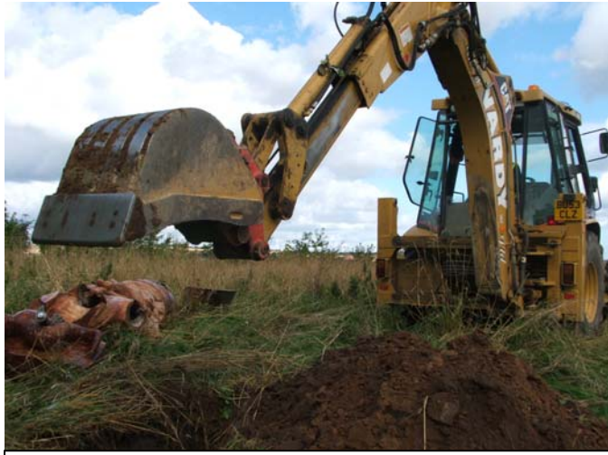
A mechanical excavator is observed as a foundation is dug for an art sculpture
